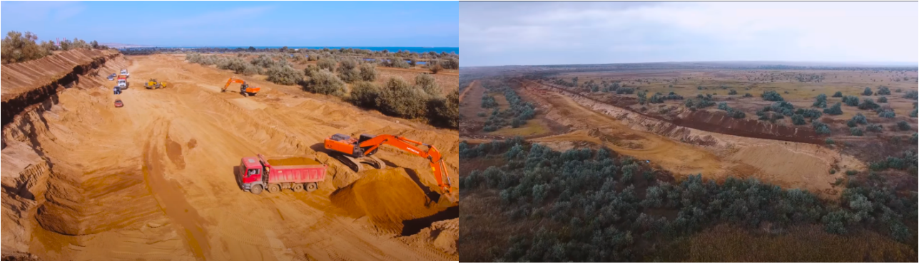
Fig. 16-17. Excavation of sand from the Nizhne-Churbassky tailings dam in 2016. Sources: Crimea Gates , Kerchnettv .
