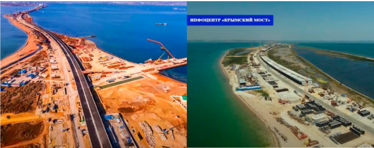
Fig. 3-4. Construction of the Crimean Bridge on Tuzla Island. Sources: Viktor Babkin-Altair Studio and KerchTV .
