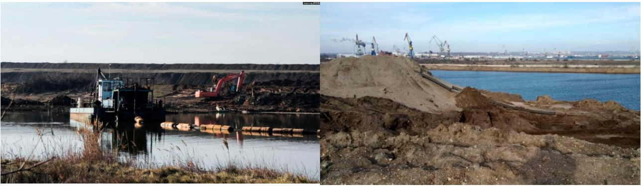
Fig. 20-21. Sand removal from the bed and banks of the bypass channel of the tailings dam with the help of a dredger in 2019. Sources: Krym.realii , Mikhail Dneprovsky (LiveJournal nordstrim).
