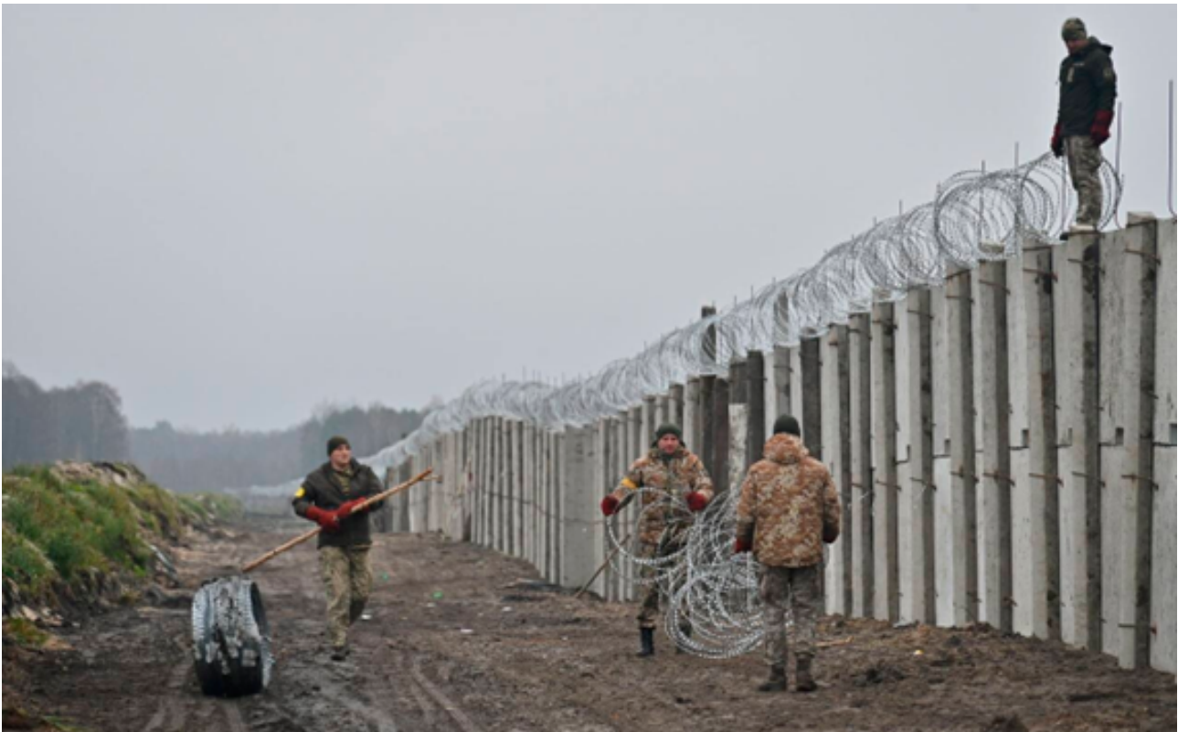
First kilometers of reinforced concrete wall appear along the Ukraine-Belarus border in 2022. This artificial barrier cannot be penetrated by small land-based animals. Source: Kirill Timoshenko / Telegram.
